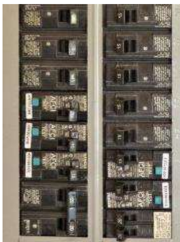
Figure 6. Breaker Box Equipped with GFI Breakers.
